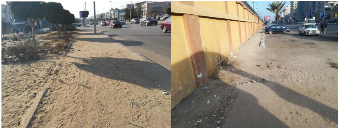
Figure 12. Poorly maintained footpaths: New Cairo (left) and Al Azhar (right).
