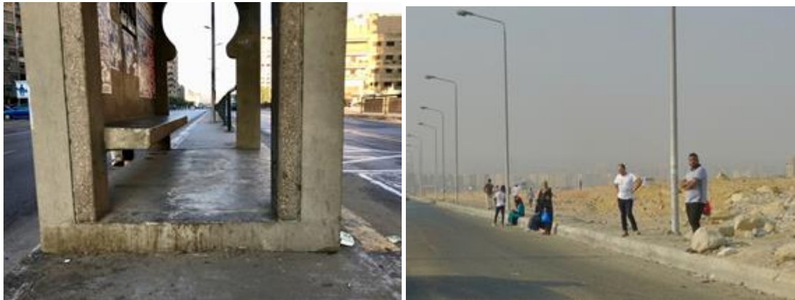
Figure 22. Recently installed bus shelters in Al Hayy Ath Thamin have a large step, compromising access for persons with disabilities (left). In the new communities like 6th of October City (right), shelters are often absent.
