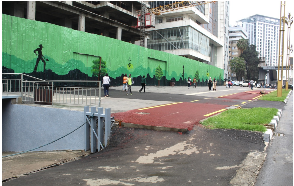
Figure 6. Disrupted cycle track at a basement parking entrance near the stadium area.
