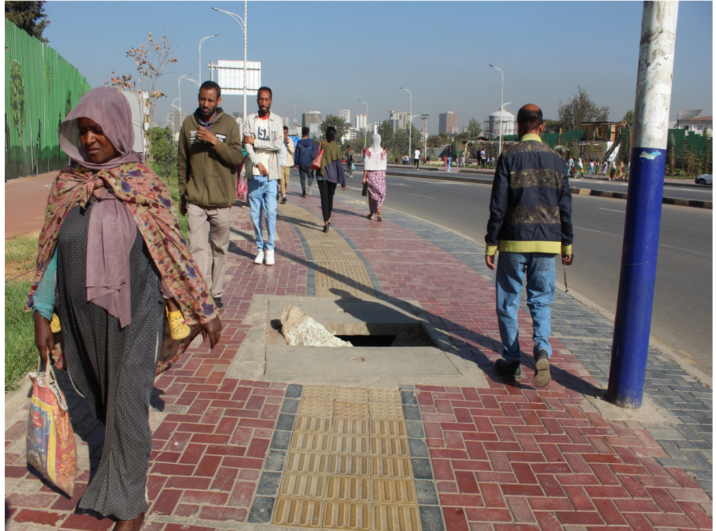
Figure 4. Discontinued tactile paving and an exposed utility hole pose serious safety risks that must be rectified.
